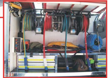
Four Electric Hose Reels after the Streamline Retrofit
